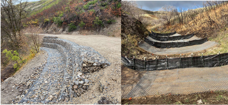
Spring Water Storm Drain
